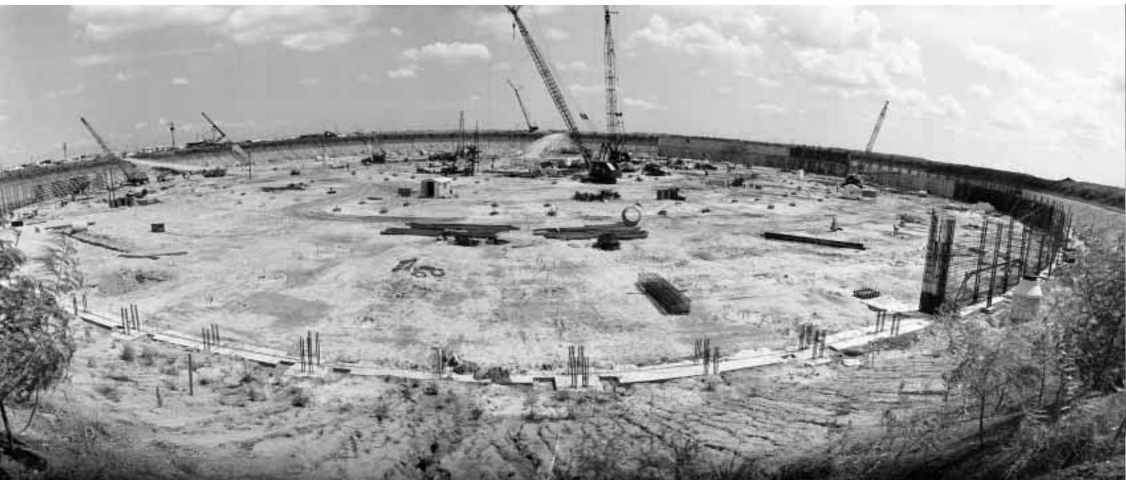
A ring of concrete and steel encircled the area to be covered by the Dome, in which many events would be played out and untold memories would be made over the next 37 years.
