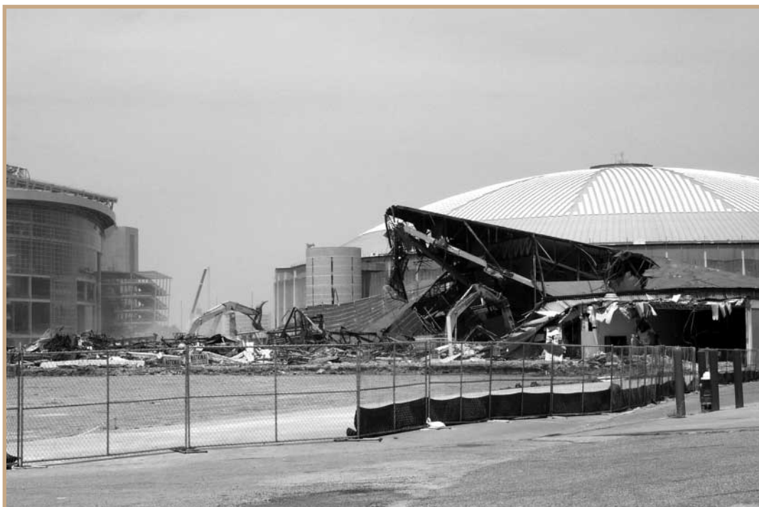
On May 1, 2002, demolition reached the rotunda of Reliant Hall, which had been the center of Houston Livestock Show activities for 37 years. The site has been paved to provide additional parking at Reliant Park.
