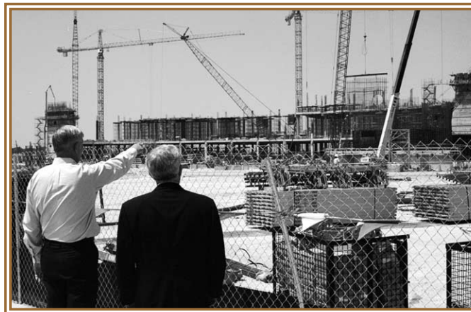
Show President P. Michael Wells and General Manager Dan Gattis survey the progress as additional levels are added to the west side of the stadium.
