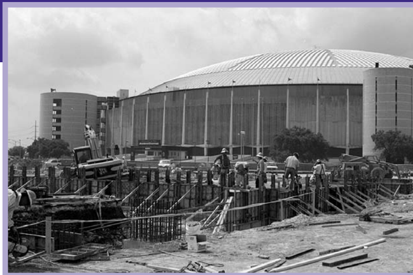
In the shadow of the Astrodome, the new RODEOHouston/NFL stadium begins to take shape. Updated photos of stadium construction are available on the Show's Web site at www.hlsr.com .
